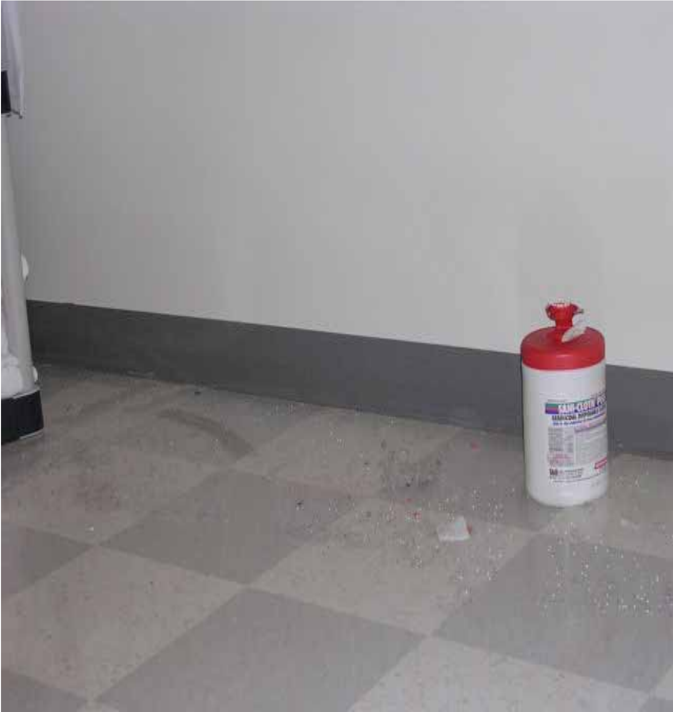
MRI Floor – Note that only the front half has been cleaned
