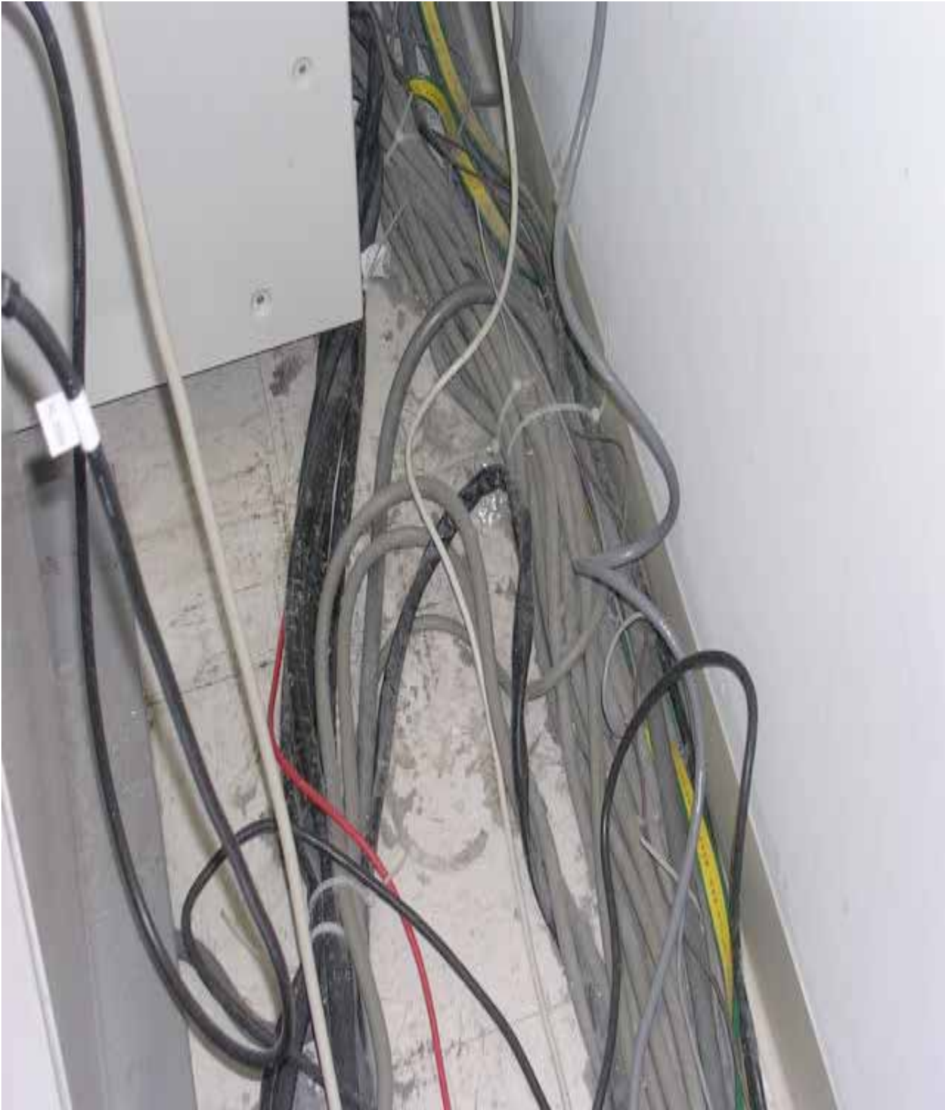
Cables in the MRI Room
