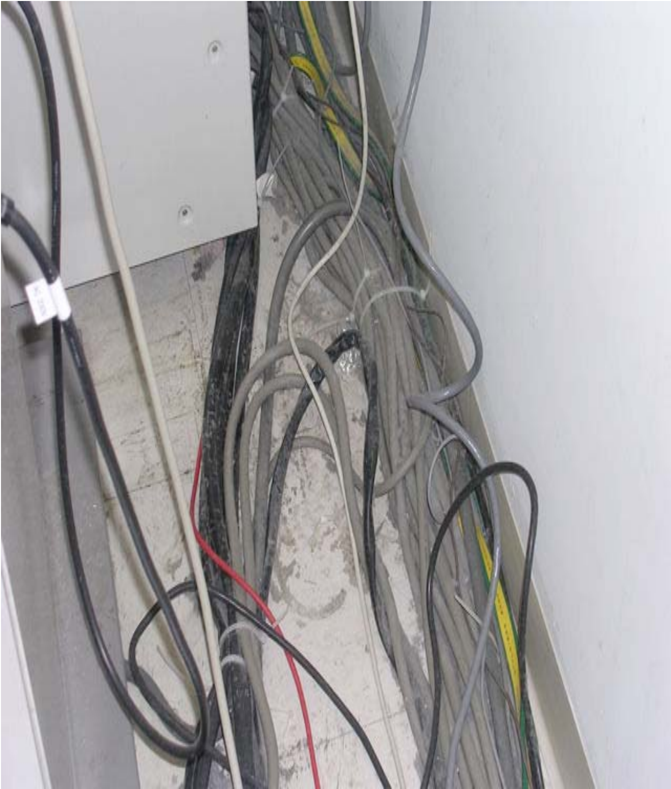
Cables in the MRI Room
